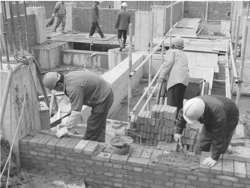
Figure 24.2 Workers laying brick to build a wall on a construction site in Colombia. Note that the workers in the back are walking across sheets of plywood that do not appear to be secured. (Photograph by Julietta Rodríguez Guzmán, Universidad El Bosque, Colombia.)
